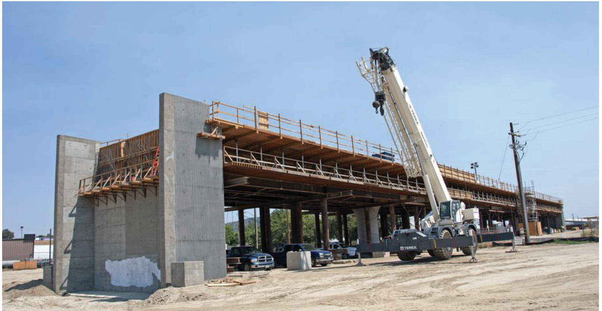
Construction of the Muscat Avenue Viaduct seen west of State Route 99 in Fresno, California.
